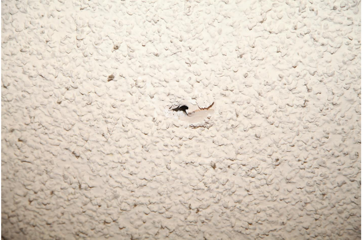
Bullet hole located in ceiling of master bedroom.
