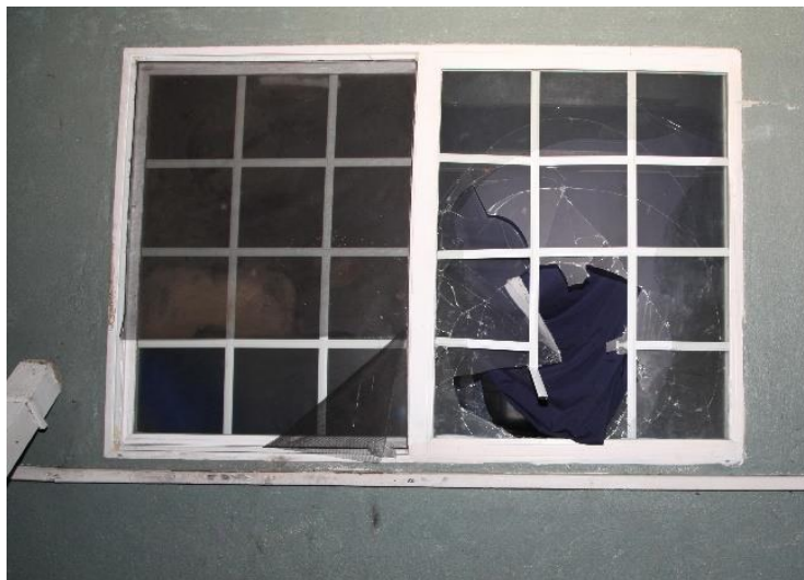
Broken front window
