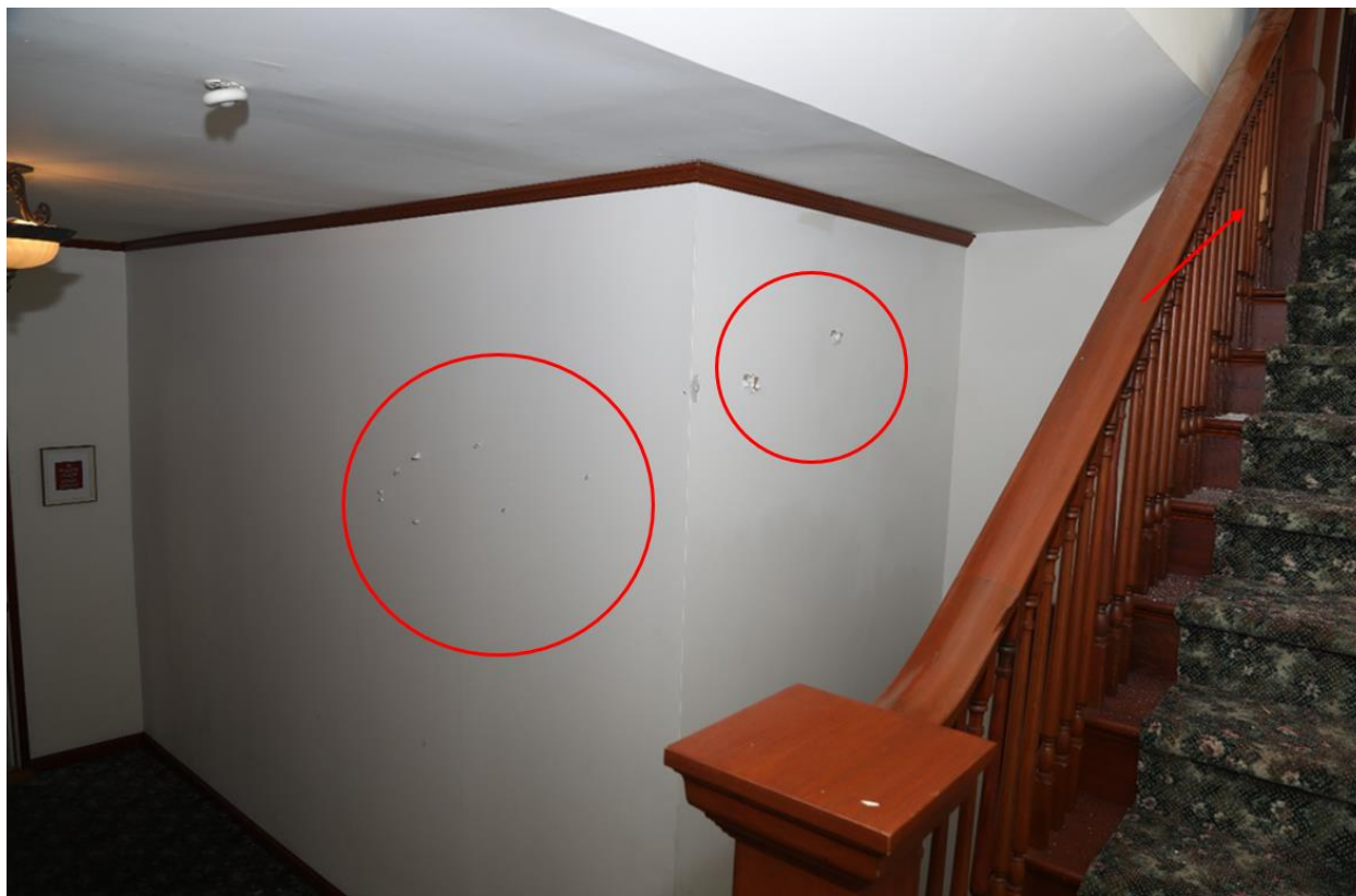
Figure 3. Entry damage on the north-facing (left) wall, and exit damage on the west-facing (right) wall caused by bullets fired from Carrillo's firearm. Damage from a bullet can also be seen on a vertical wood rail near the top of the stairs.
