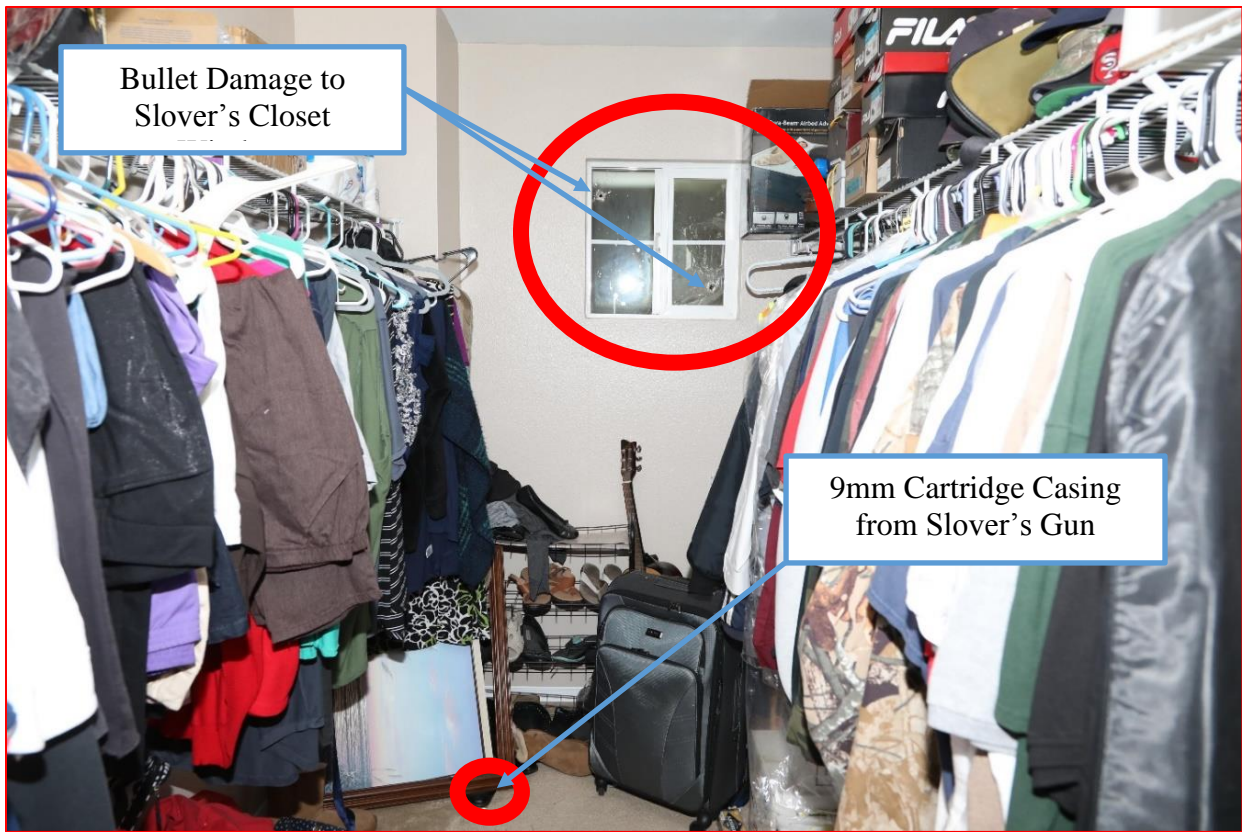
Figure 2- Photo of interior of Slover's closet showing bullet damage to the window and a 9mm cartridge casing on the floor.
