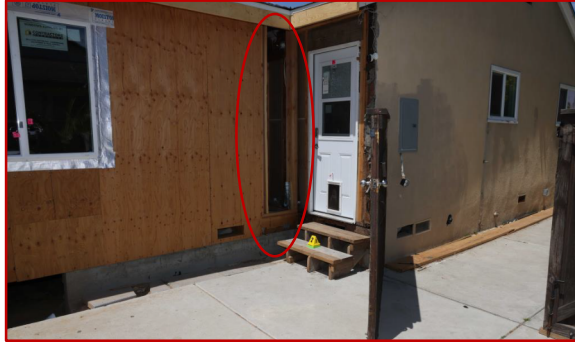
Figure 4: Gap in Front House from which Sanchez Emerged (Circled)
