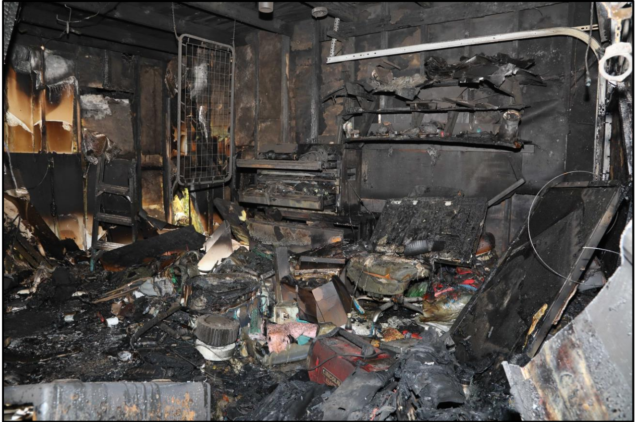
Figure 16: Main garage area, extensively fire damaged and littered with debris
