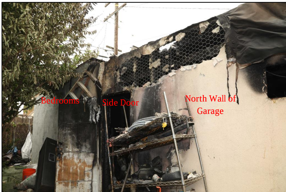
Figure 4: Fire-damaged wall of Herrera's garage, viewed from the backyard
