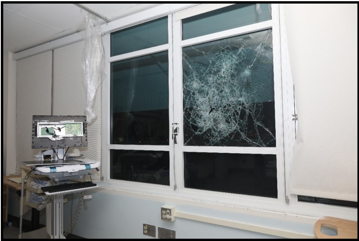
Figure 4: Damaged window and computer monitor inside room 4E-12.
