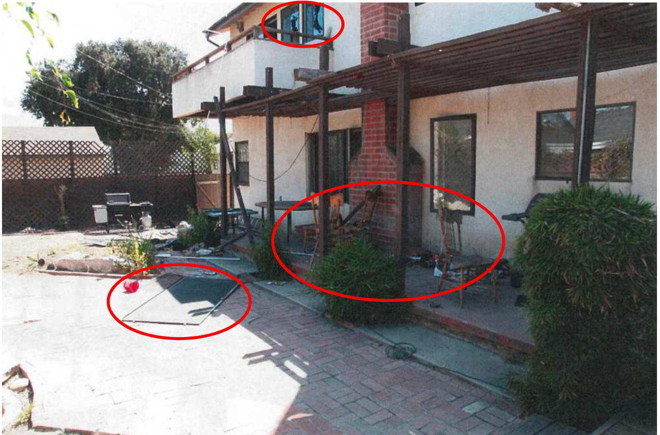
Backyard with Screen on Ground, Broken Furniture and Broken Windows
