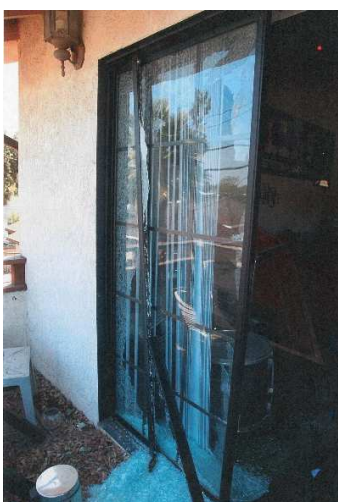
Shattered Sliding Glass Door to Master Bedroom
